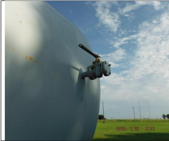
Valve bolted to flange
