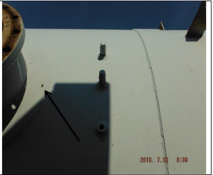
Repad plugged with threaded plug
