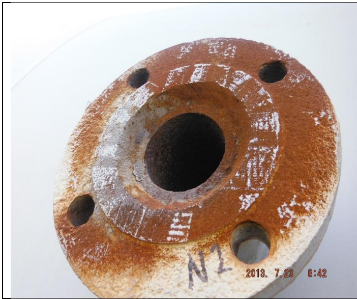
Corroded Flange Face
