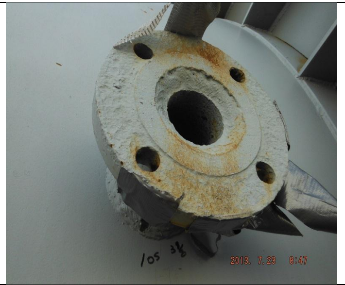
Corroded Flange Face
